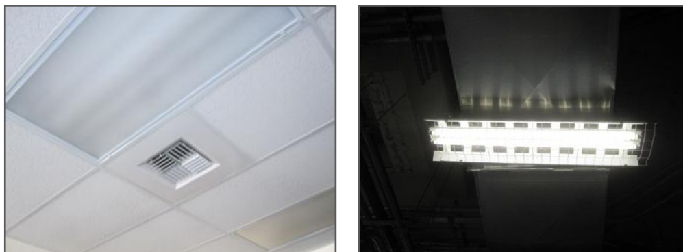
Typical light fixtures at TMWRF: Administration Building (left); Nitrification Pump Station (right)
