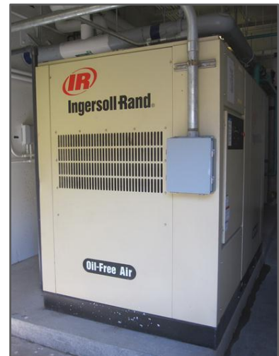
Ingersoll-Rand air compressor for DAFT process.
