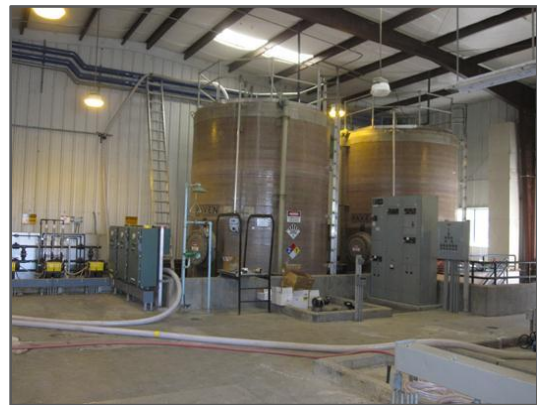
Aluminum bisulfate tanks
