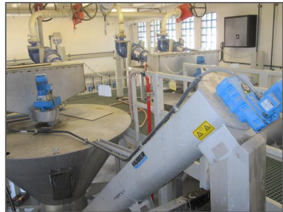
Grit separators in the Grit Removal Building
