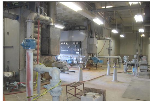
Sludge heaters 3 and 4 in Digester Control Building No. 1
