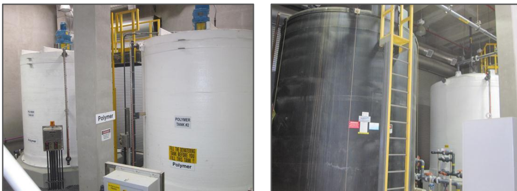
Polymer (left) and ferric chloride (right) tanks in Chemical Building No. 2
