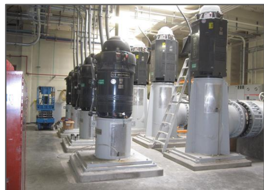
Influent and effluent pumps at the Nitrification Pump Station.
