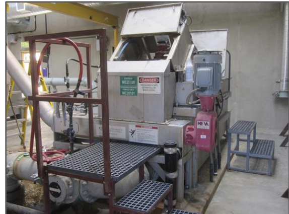
Sludge screener at the Primary Sludge Screening Building
