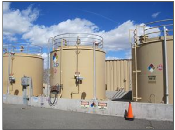
Methanol tanks for the denitrification process.
