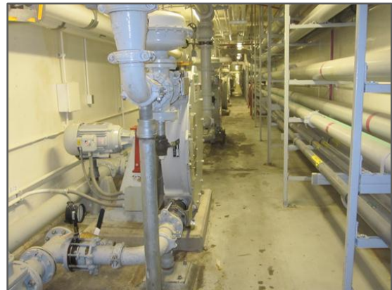
Gallery C with the row of sludge and scum pumps for the primary sedimentation tanks.
