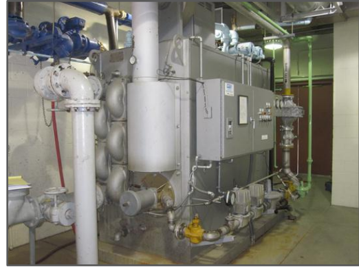
Sludge heater 5 at Digester Control Building No. 2.
