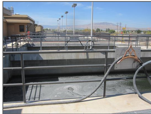
Filter facility for post-aeration effluent
