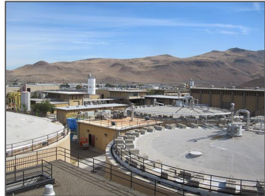
Methane digesters with digester gas collectors on the top.
