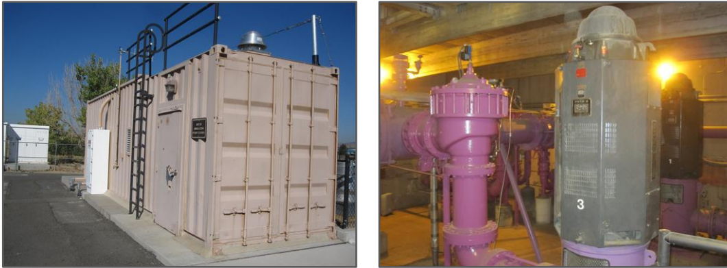
Reuse irrigation pump station (left); Underground pump room (right)
