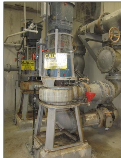
RAS pumps 1 C-1 and 1 C-2 in Gallery A.
