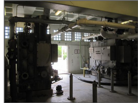
Sludge heaters numbers one and two in Digester Control Building No. 3
