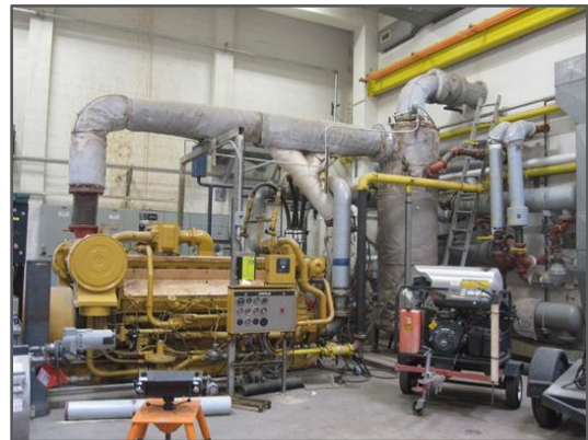
Existing cogeneration system (not used).
