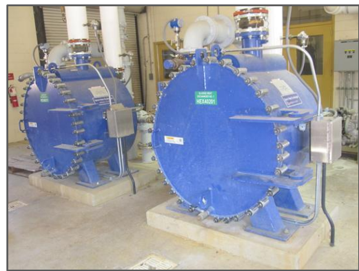
Sludge heat exchangers numbers one and two at Digester Control Building No. 4.
