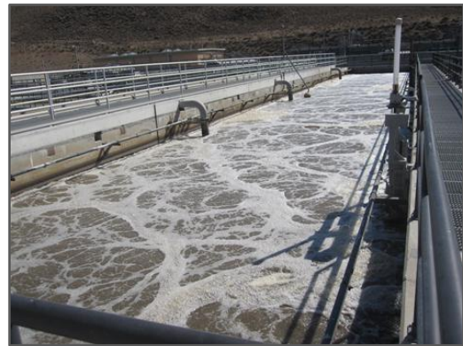
Aeration tank at TMWRf
