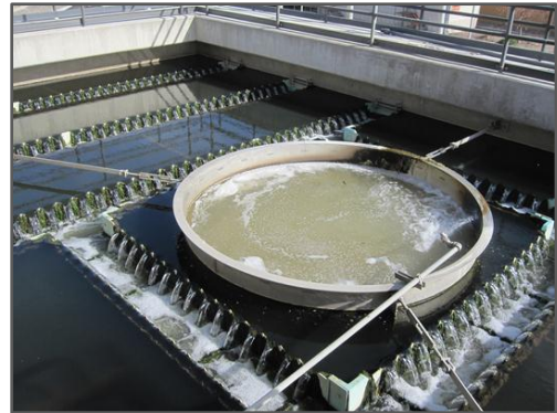
One of the four denitrification tank.
